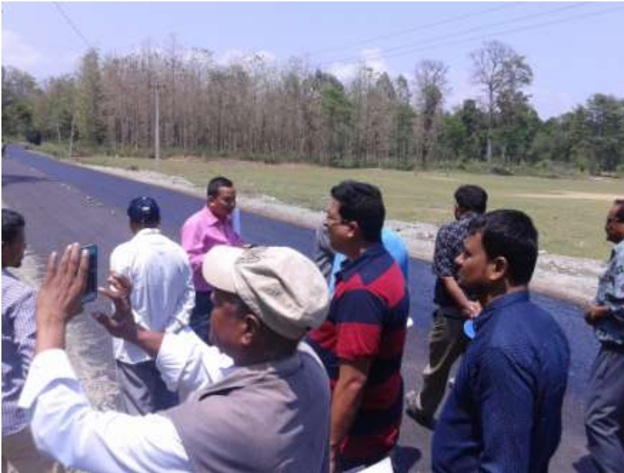
Jt. Monitoring of K-K Road by DTICC Members (LDO/DTO/Political leaders/DTL /Imp. Team/Contractor) after Prime Coat
